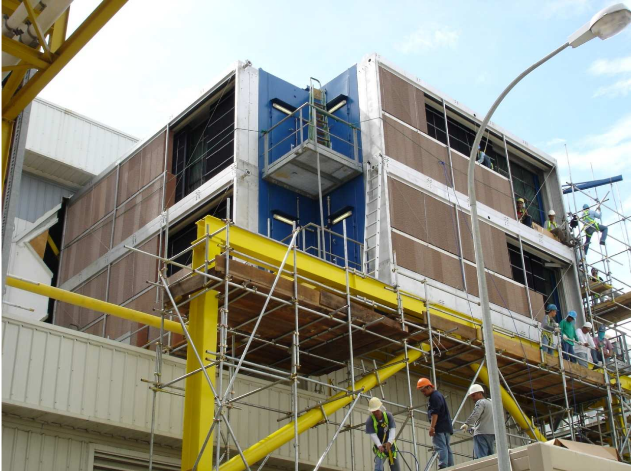
Siemens V 94 in Santa Rita/ Philippines
