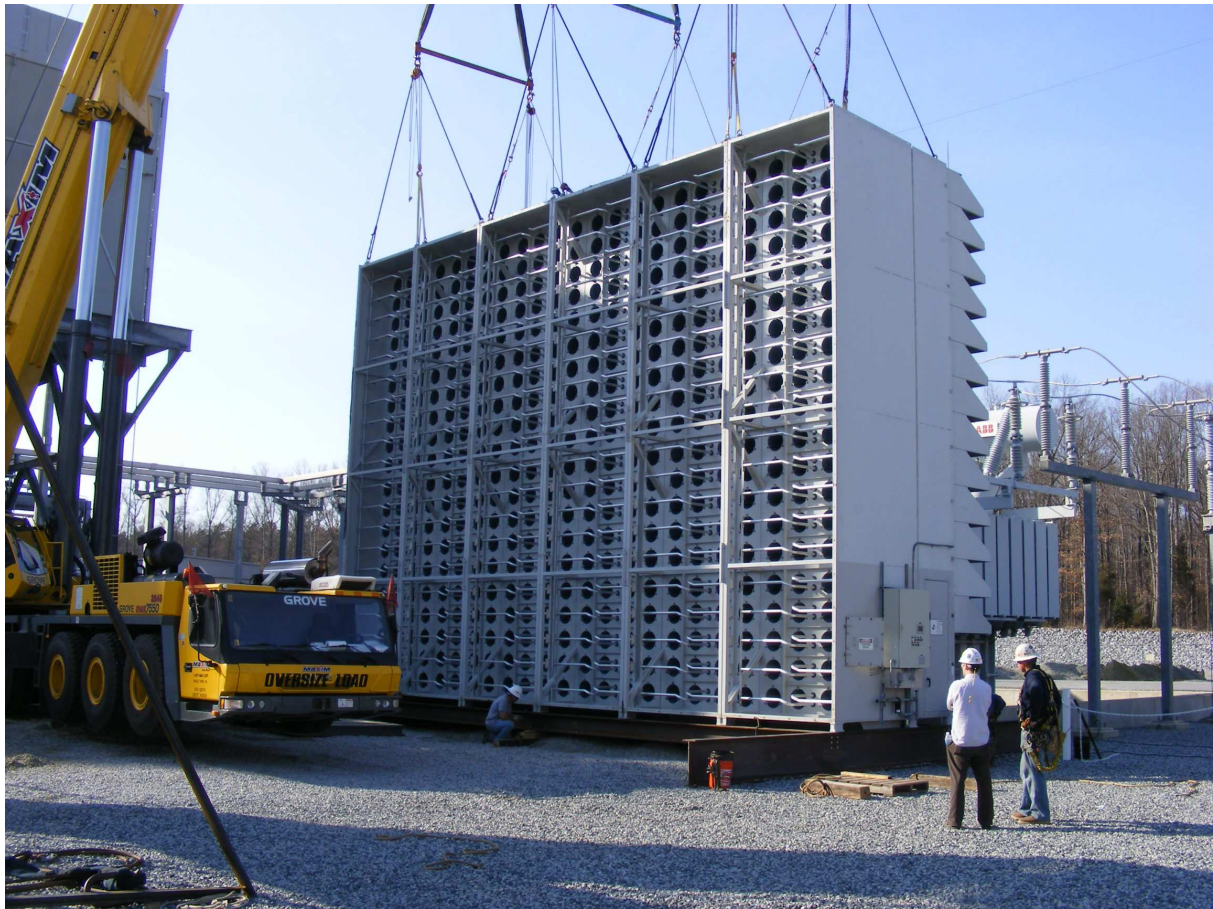
pulsefilter housing on „park position“
