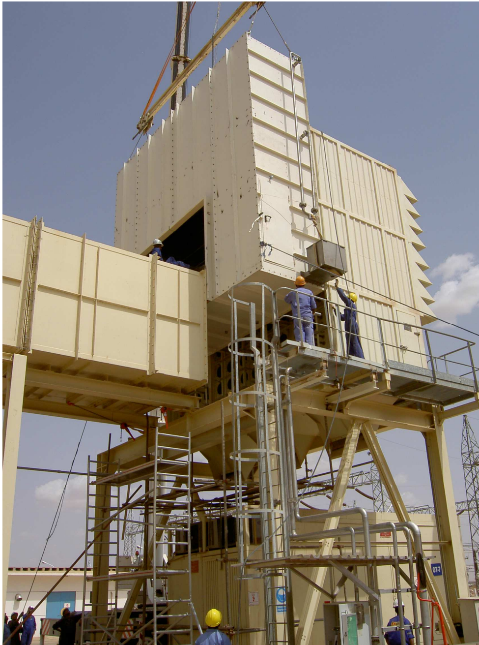
Frame 6 with new transition duct incorporating the evapcooler also
